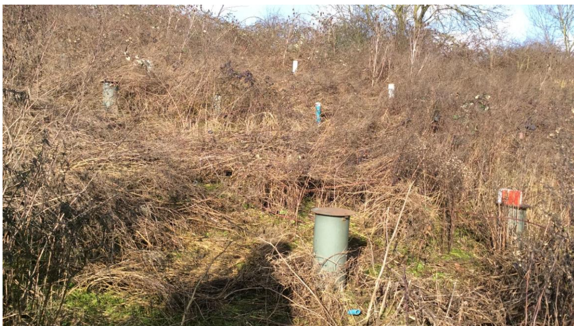
Figure 2: Heavily vegetated FRS slope. Raised installation covers rotated between 3° and 5° to the west
